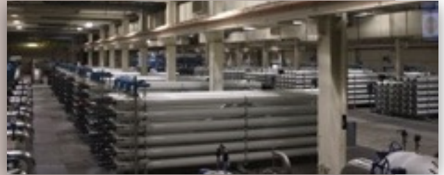
rows of various sizes of filters at the Water Campus
